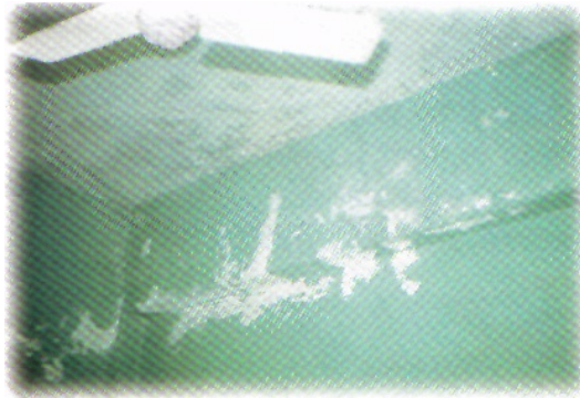
Fig.9. Leakage from roof slab
