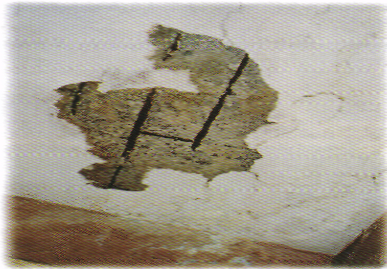
Fig.4. Corrosion of steel and spalling of concrete due to ingress of moisture
