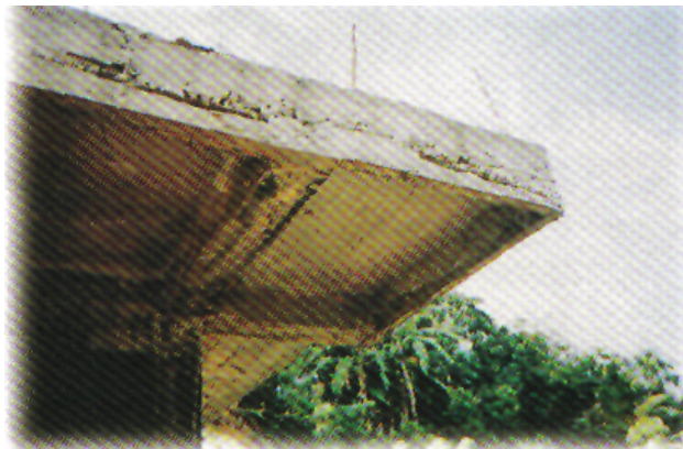
Fig. 7. Cantilever canopy showing honeycombing
