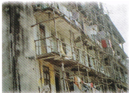
Fig.8. Badly deteriorated slender cantilever balcony slabs.
