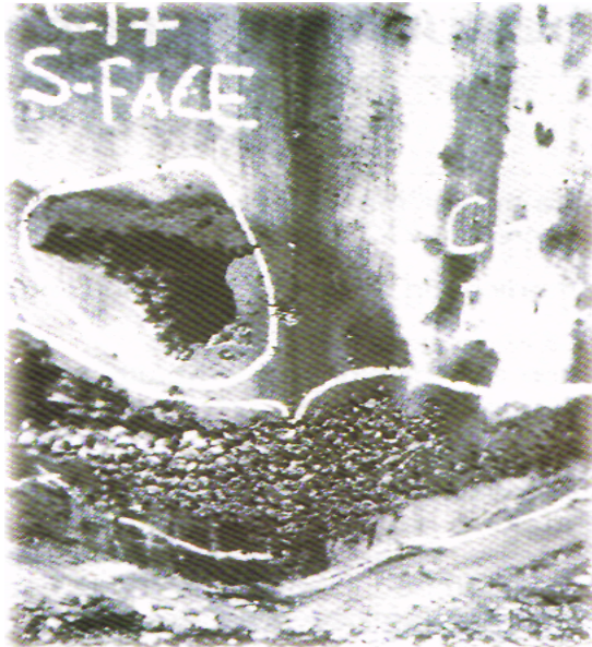
Fig. 2. Honeycombs at the foot of a RCC column
