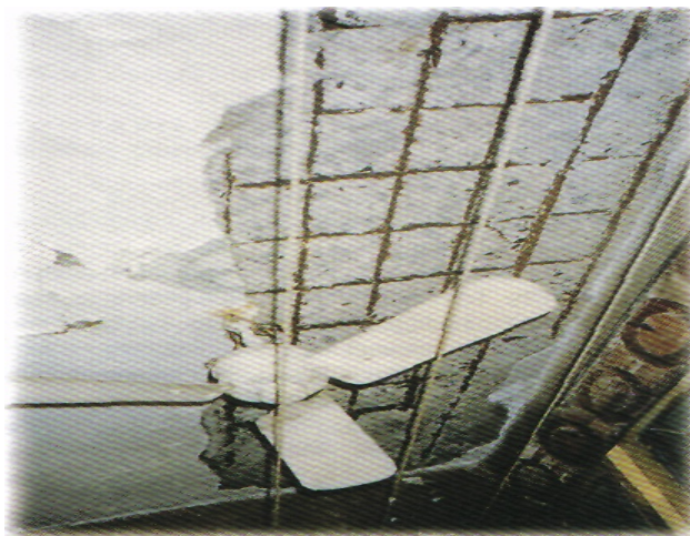
Fig.10. Spalled concrete due to corrosion of steel
