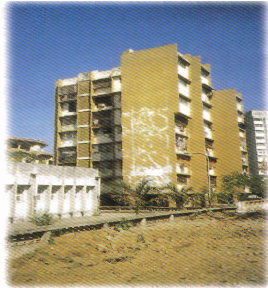
Fig. 3 Wide cracks on concrete wall and on plaster
