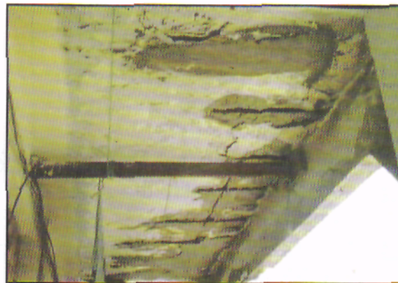
Fig. 5. Corrosion of steel in a canopy
