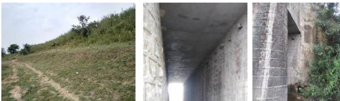
Figure 3: Canal outer face & Culvert condition in same stretch after B G Mlining.
