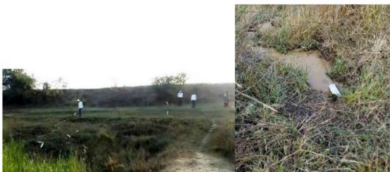
Figure 2: Canal outer face Seepage in same stretch before BGM lining.
