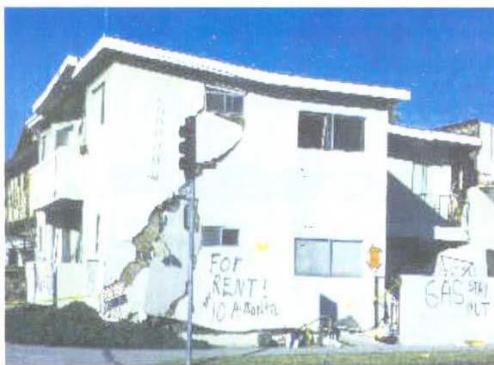
Figure 3: Cracks in Masonary Wall
