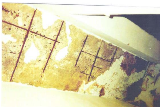
Figure 7: Corrosion in the RC slab (lack of control on the cover)
