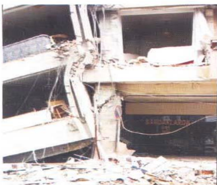
Figure 5: Tilting of Columns
