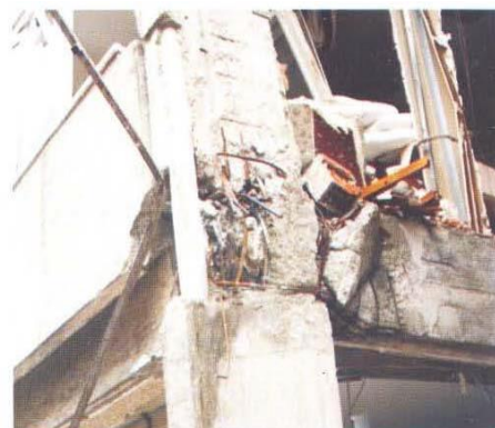
Figure 6: failure in column beam joint
