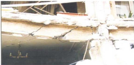
Figure 1: Cracks in RC beams
