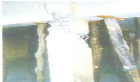
Figure 2: Cracks in Columns
