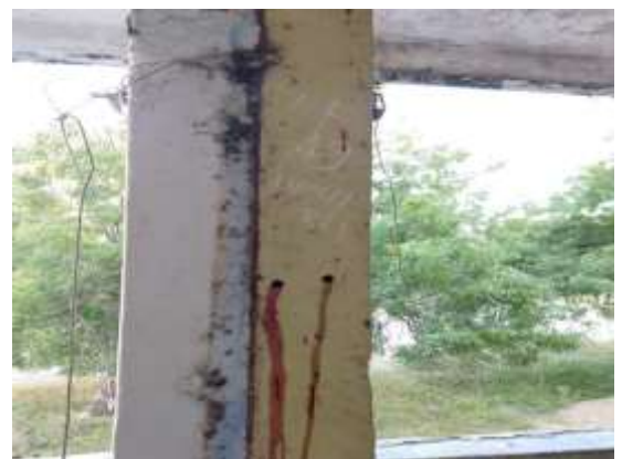
Fig.4.5.1 Depth of Carbonation
