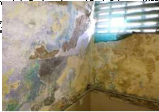
Fig.4.1.4 Seepage in the walls
