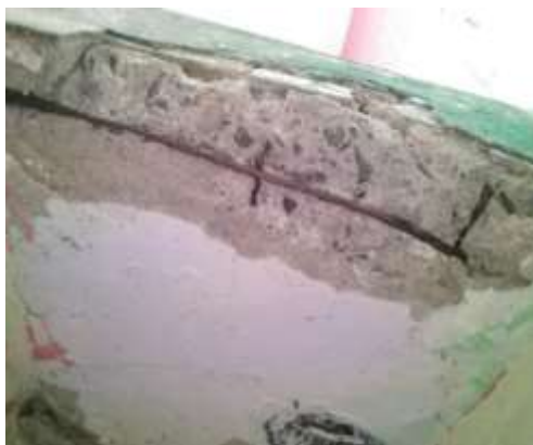
Fig.4.1.1 Reinforcement Exposed in
