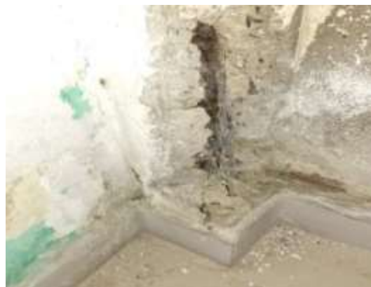
Fig.4.1.2 Deterioration of Column
