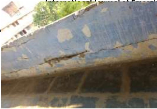
Fig.4.1.3 Cracks in the Parapet Wall
