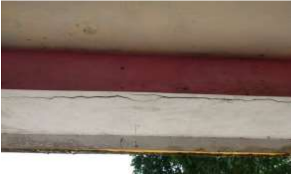
Fig. 2.1.5 Crack in beam
