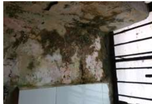
Fig. 2.1.6 Seepage and vegetation on wall
