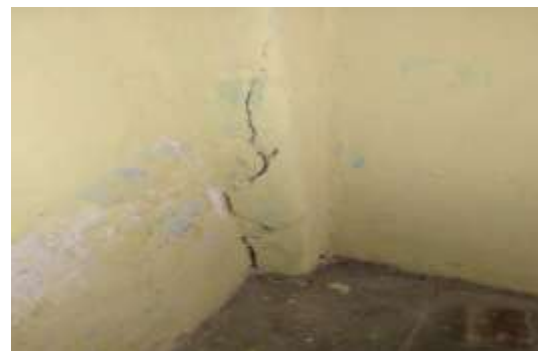
Fig.2.1.2. Cracks in Columns
