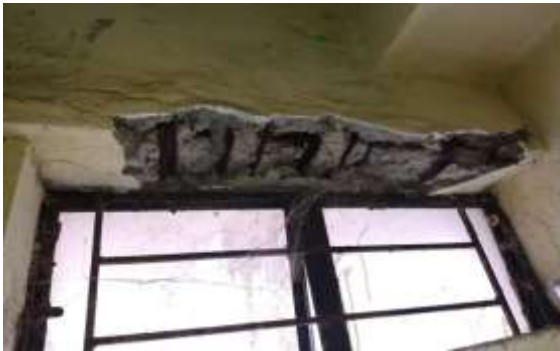
Fig. 2.1.1 Reinforcement exposed in Lintel
