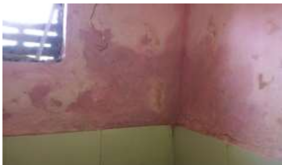
Fig.2.1.3. Seepage in walls
